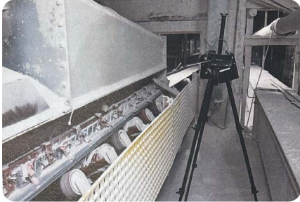
Setup of the measuring instruments after installation of the AirScrape® system.
