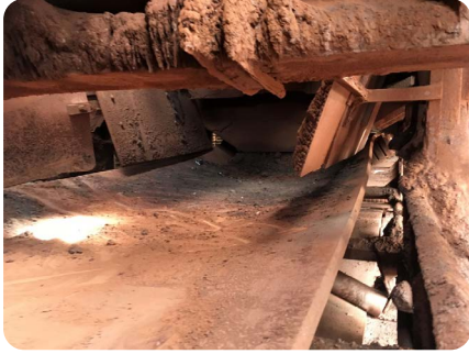
The transfer point prior to installation: material discharge in all directions due to insufficient sealing.
